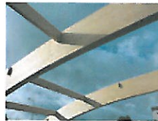
The Limitless jointing system is barely visible on glulam beams
